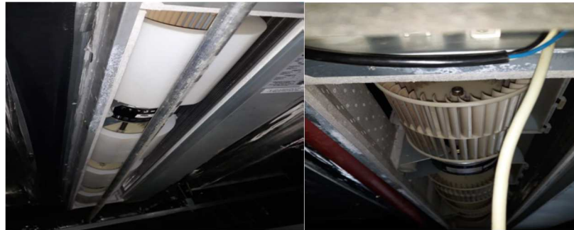
Figura 2 – Turbinas dos fan coils
